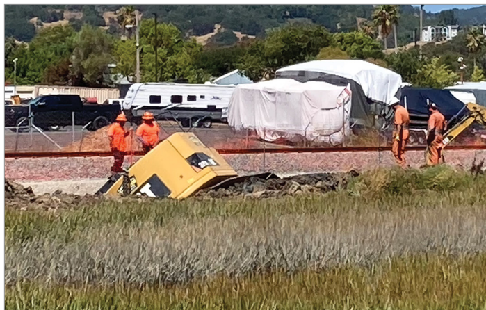
Heavy equipment stuck in marsh at SMART multi-use path construction site on Gallinas Creek
